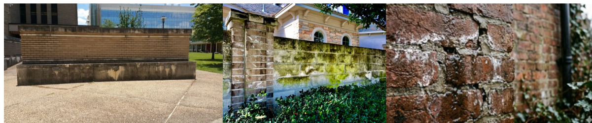
Figure 2: Damaged walls of different brick types that show efflorescence, mold, mildew, and water damage through delamination and loss of concrete. Photo credit S. Curran.
