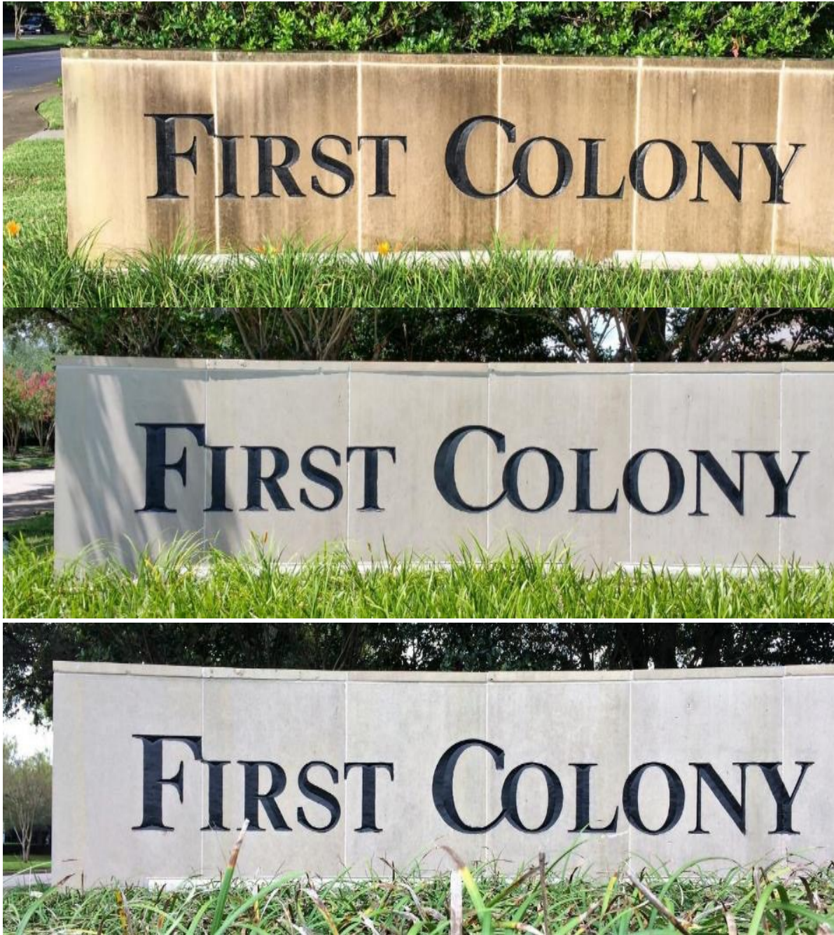
Figure 8: These monument signs were being constantly damaged by mold, mildew, water degradation, and constant pressure washing. Treatment with a penetrating cross-sealing silicon-based coating maintains the properties for up to seven years, 4 to 6 years' improvement on current offerings from old paint companies.
