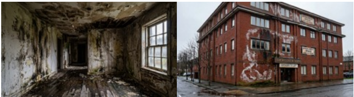
Figure 12: This is what will happen both on the interior and exterior of buildings simply caused by water damage, leading to mold and mildew, as well as efflorescence (white color) and physical delamination of the walls.
