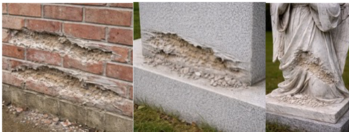
Figure 10: The damage that can be caused by poorly skilled pressure washer technicians.
