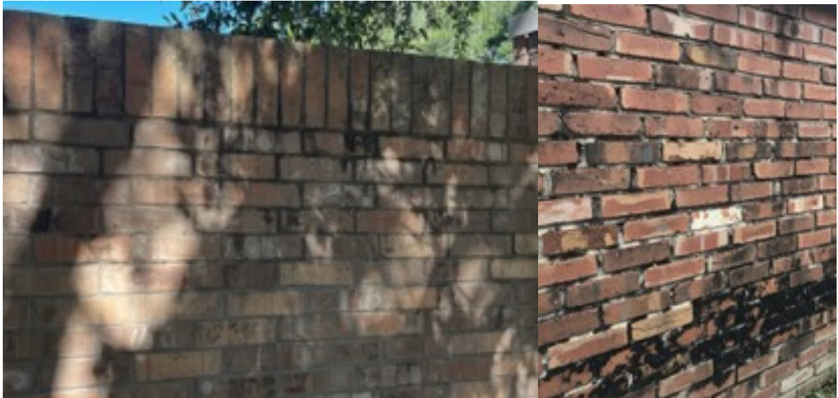
Figure 6: Degradation of walls through organic matter such as bacteria, lichen, mold, and mildew. Mold and mildew on brick walls at New Territory, Sugarland in the greater Houston area. This work will last up to 7 years before signs of growth and water damage will appear. The HOA runs the community operations that keeps the environment in such a manner that curb appeal is maintained because the whole appearance of the area is well managed.
