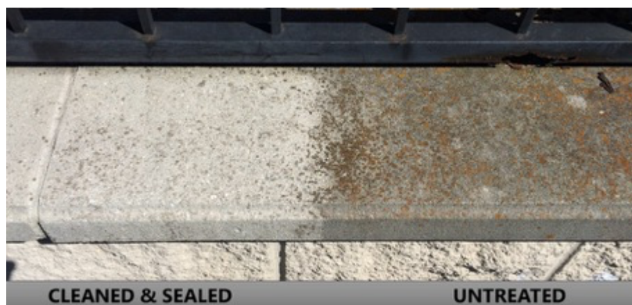
Figure 1. Comparison of cleaned and treated masonry (left) and normal untreated stone (right), with the untreated stone showing a prominence of rust from metal railing leaching through the masonry.
