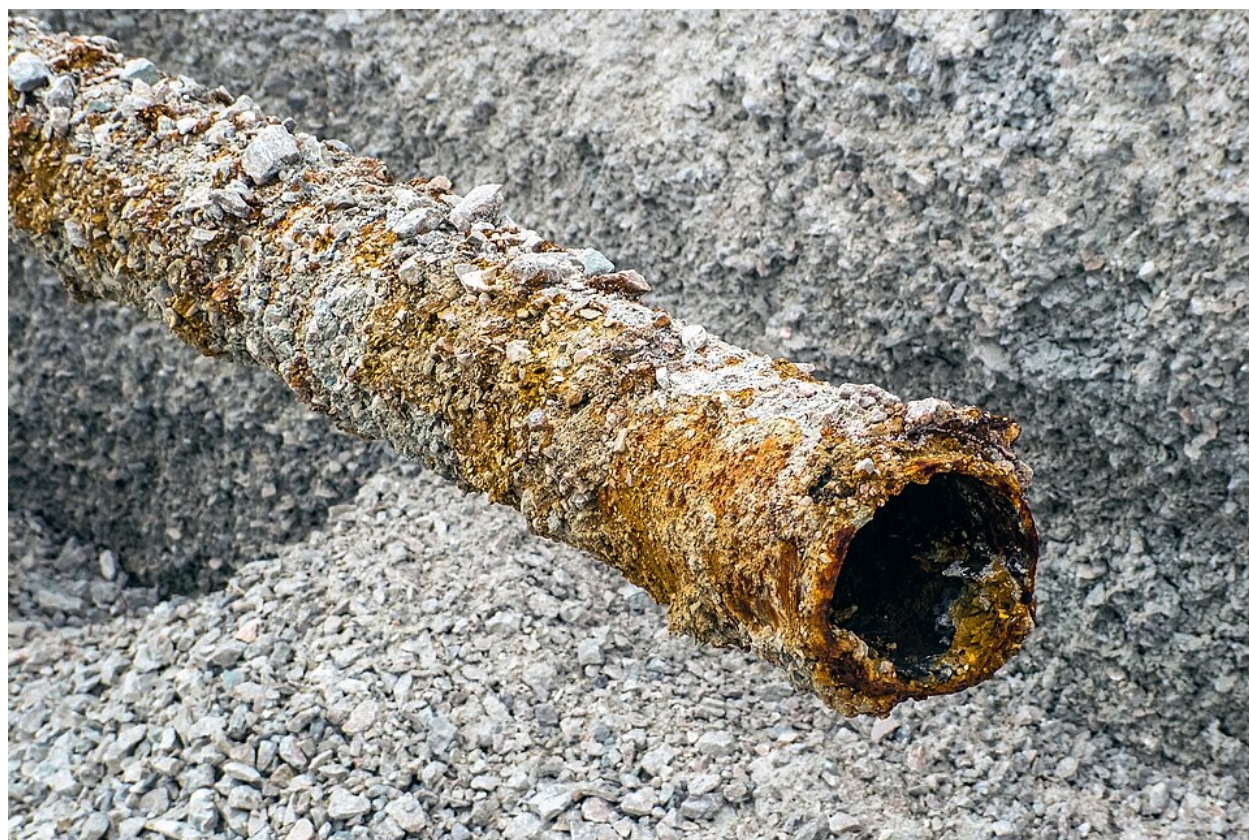
Figure 11. Heavily degraded by water damage, corroded pipes stand near a pier in the factory area of the abandoned limestone quarry on Furilden, Gotland, Sweden. Source: Wikipedia Commons
